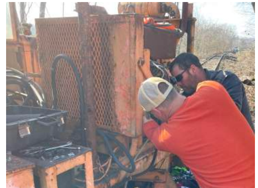
Chief Mechanical Officer, Caelib Qualkenbush (orange shirt), and mechanic, Dave Knieriem work to replace a broken compressor on the tie crane.
