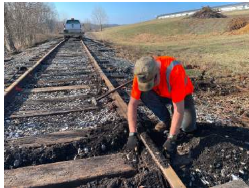
Steve Hobson places a tie plate between a newly installed tie and the foot of the rail in preparation for spiking the rail.
