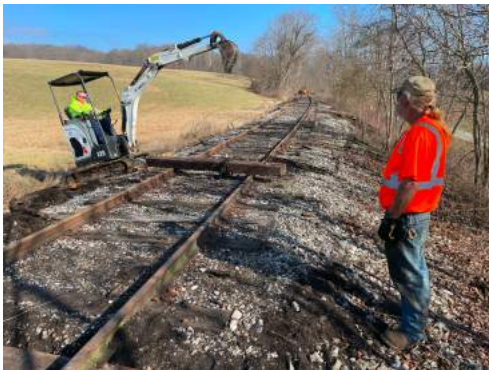
Track Foreman trainee, Bobby Tincher, and long-time lead track maintainer, Steve Hobson, work to insert relay ties near Crystal at MP 66.5.
