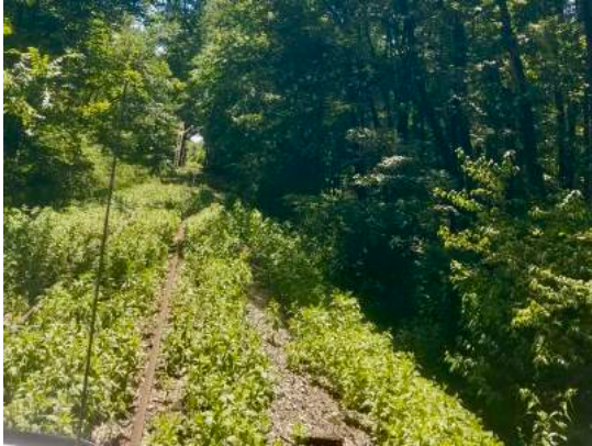
Overgrown weeds are shown nearly covering the tracks as seen during a hi-rail inspection. Photo taken by Brian Small.
