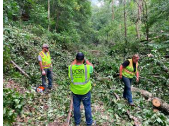
Staff members Kaleb Webster, Emma Albright, and Shane Denu are working to clear limbs and branches from the tracks around MP 74.
